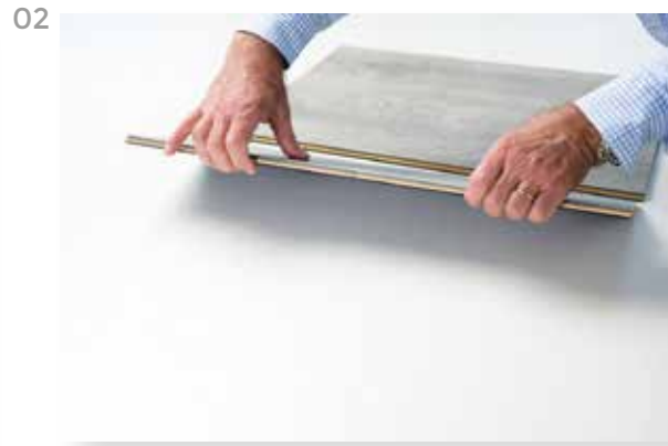
Grab the planks with both hands and gently lift at the same time until the planks disengage
